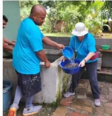
Charles (Jr.) Ashford and Nikki Connell working on cleaning the rocks that go into the water filtration system at the school.
