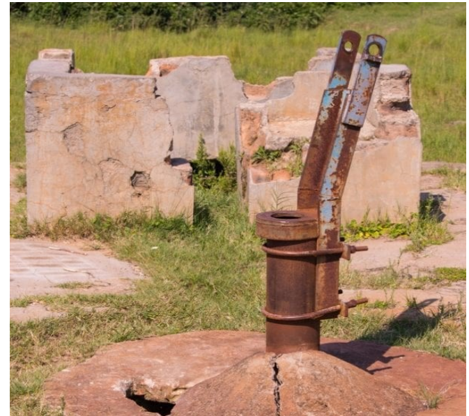
Nigeria - abandoned water well after 5 years due to lack of community maintenance
