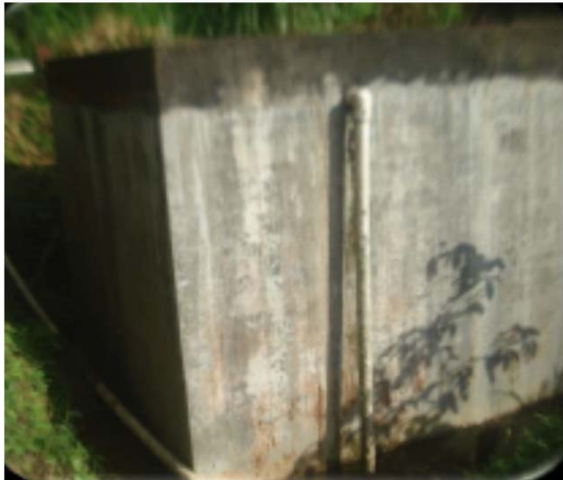
Current Storage Tank
