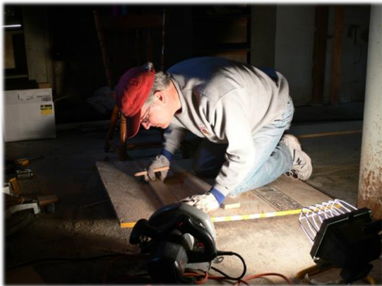
2008: John “Buckeye” Keough building a basement staircase at a Clean Sweep project.
